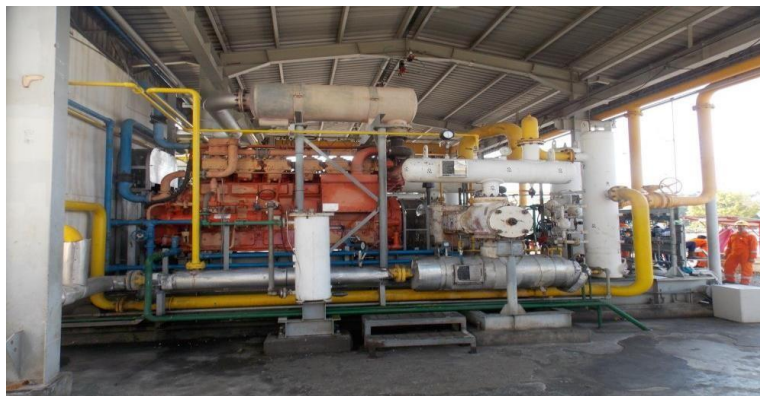
Gambar 8 Kompresor CP-9600 di Central Processing Area
