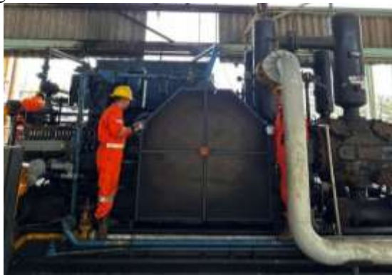
Gambar 1. Unit Gas Compressor DPC-360
